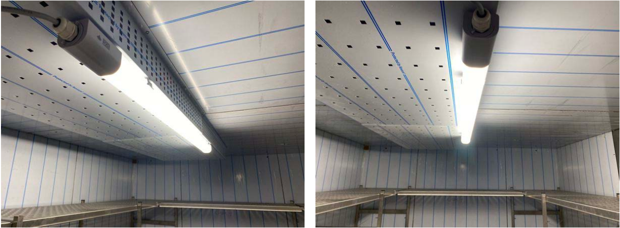
Figure 49: View of installed light
