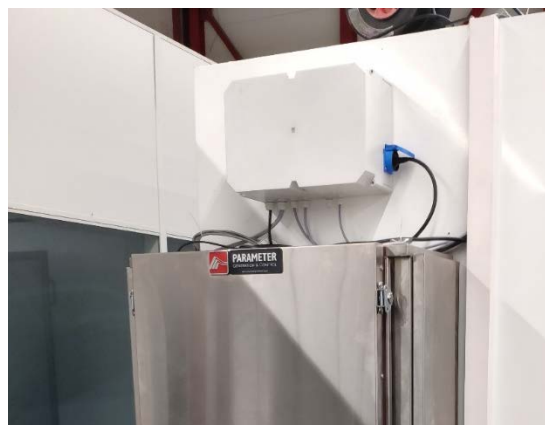
Figure 62: Connection box (blue) of the junction box
