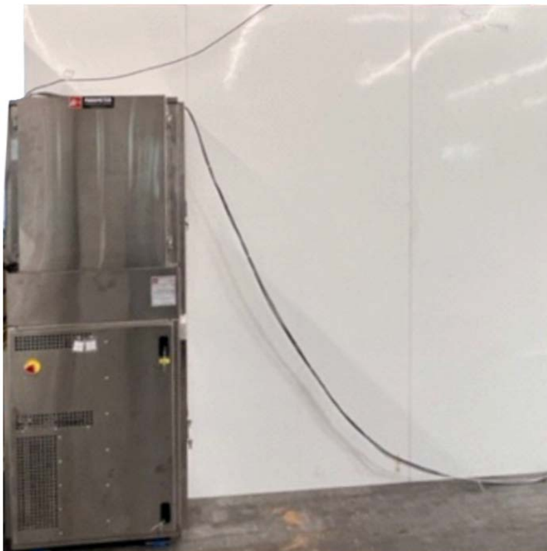
Figure 29: Position of the conditioner at the WIC chamber
